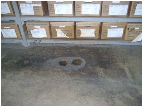
Figure 3 Water stains on the floor from roof leakage.
