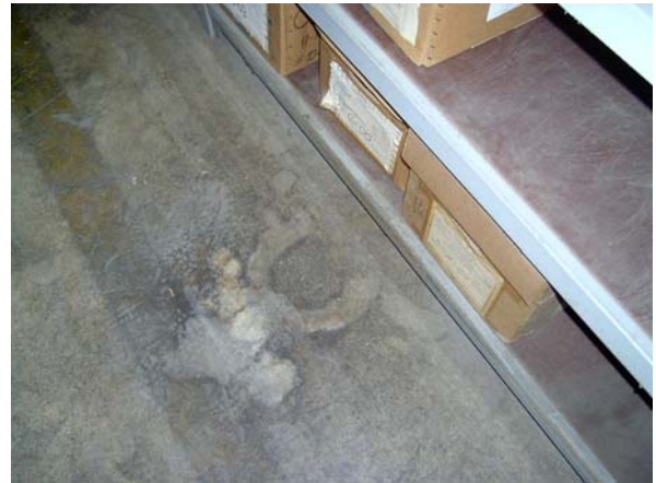
Figure 4 Water stains on the floor from roof leakage.
