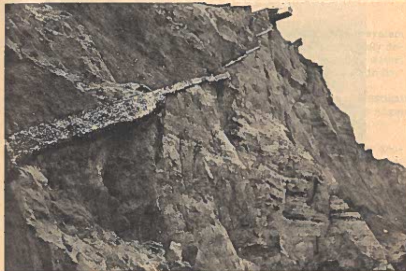
FIG. 19.—LEFT (WEST) SIDE OF CREVASSE, BALDWIN HILLS RESERVOIR
