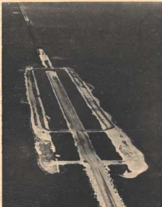
FIG. 14.—AERIAL VIEW OF RECONSTRUCTION OF "MIDLAKE FAILURE"
