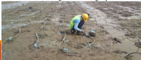
Flexible pipe system connecting to vacuum pump
